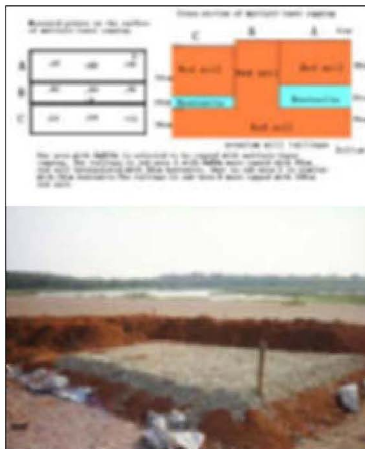
Fig. III-14. The structure to (top right) and placement (bottom) of the multiple-layer capping, and distribution of measurement points (top left) at the Erquier uranium mill tailing impoundment.
